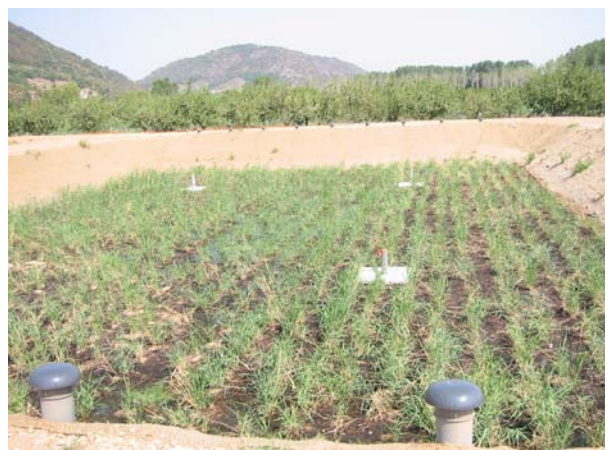
Sludge treatment reed beds
